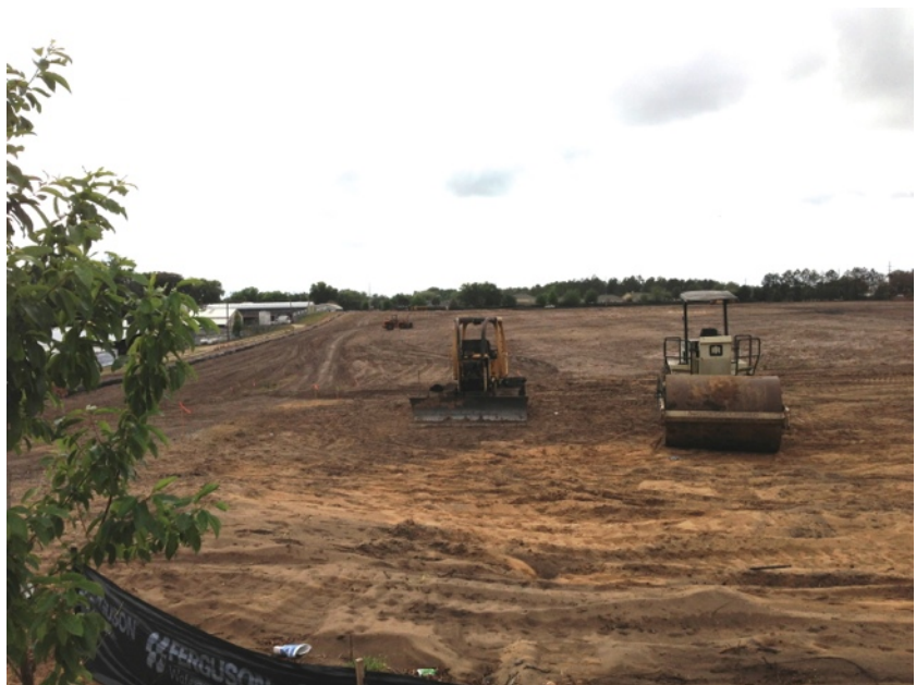
This is a photo of the cleared land beyond the end of Dunn Blvd. There will be 52 homes build there soon. Dunn Blvd will be continued to Binion Rd. See more photos in the "Photos" menu on the Home Page
